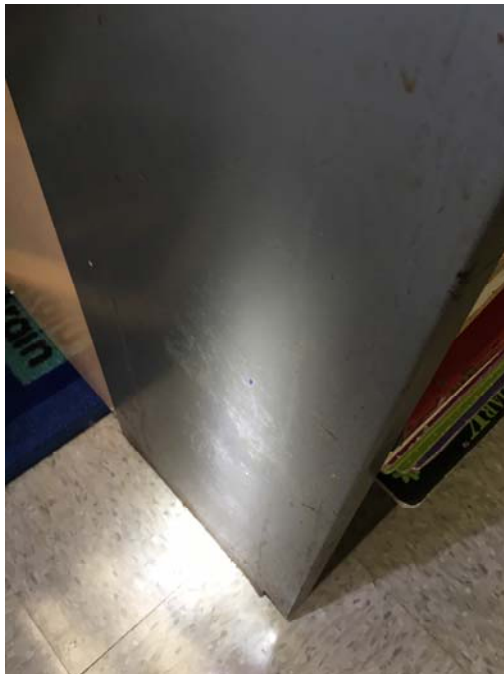
Photo 12 – Kindergarten Room 1 Mold growth was observed on the metal storage cabinet.
