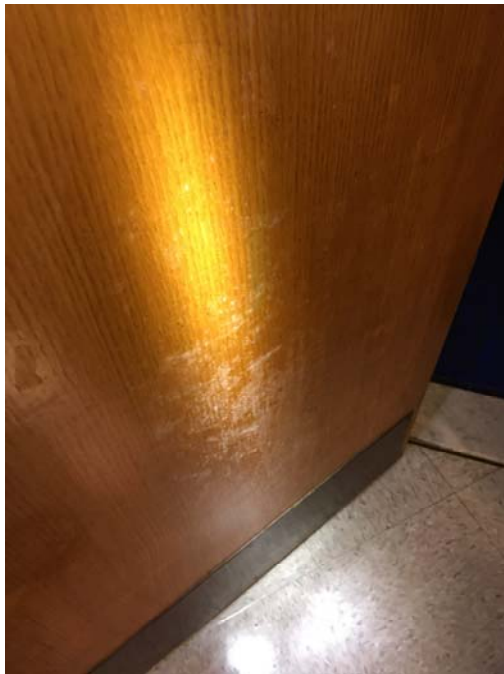
Photo 8 – Kindergarten Room 1 Mold growth was observed on the wooden door and metal frame.
