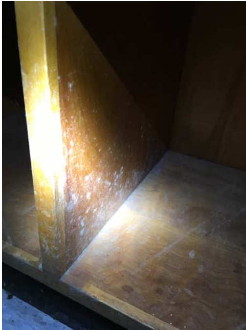
Photo 21 – Kindergarten Room 2 Mold growth was observed on the built-in wooden cabinetry and coat cubby.
