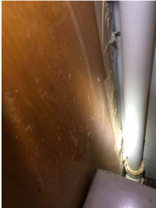
Photo 11– Kindergarten Room 1 Mold growth was observed on the wooden built-in cabinetry and coat cubby.
