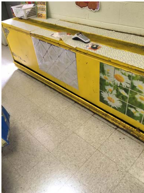
Photo 34 – Kindergarten Room 3 The return air tray was not seated properly and no air filters were observed inside this unit.
