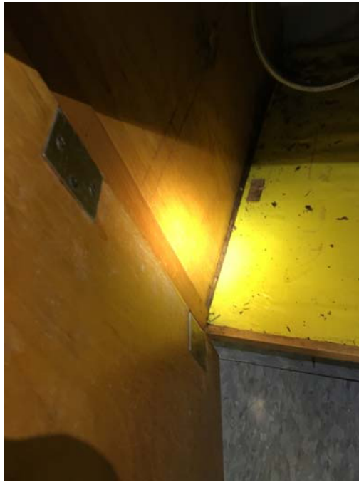
Photo 25 – Kindergarten Room 2 Mold growth was observed on the sink cabinet.
