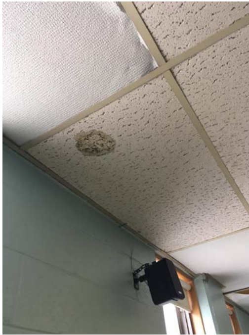
Photo 23 – Kindergarten Room 2 Mold growth was observed on a ceiling tile.
