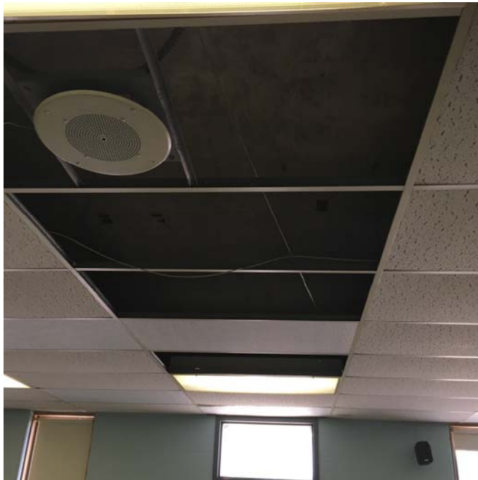
Photo 13 – Kindergarten Room 2 Missing ceiling tiles were observed.
