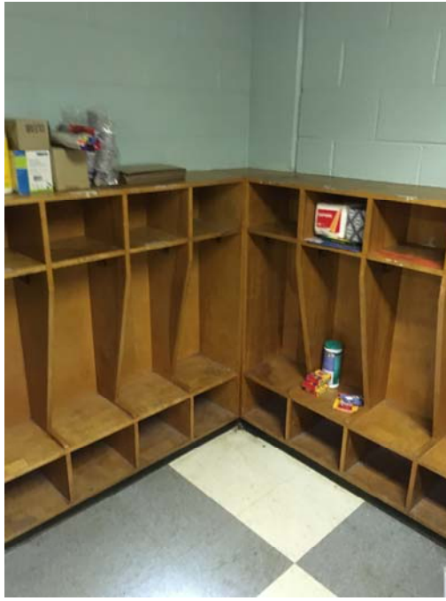
Photo 19 – Kindergarten Room 2 Mold growth was observed on the built-in wooden cabinetry and coat cubby.
