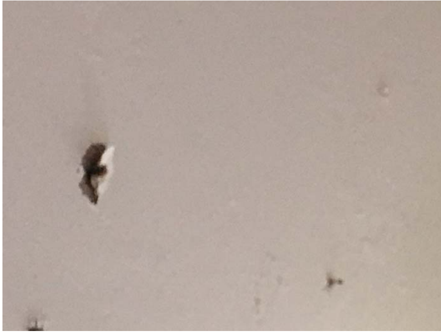
Photo 3 – Kindergarten Room 1 Small sections of spalling concrete ceiling were observed on the ceiling.
