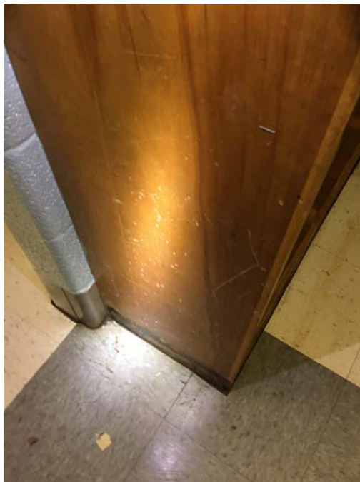
Photo 18 – Kindergarten Room 2 Mold growth was observed on the built-in wooden cabinetry and coat cubby.
