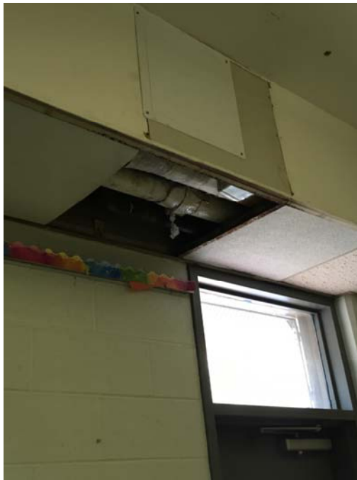
Photo 4 – Kindergarten Room 1 A missing ceiling tile and condensate was dripping from the ceiling. Wet fiberglass pipe insulation was observed above the suspended ceiling.
