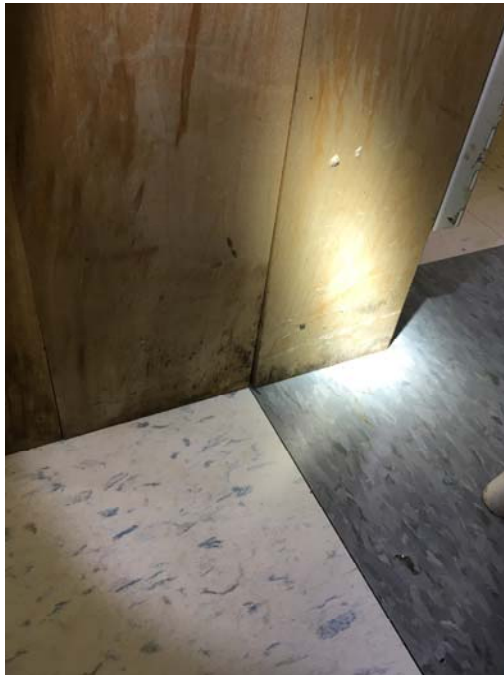
Photo 24 – Kindergarten Room 2 Mold growth was observed on cabinetry.
