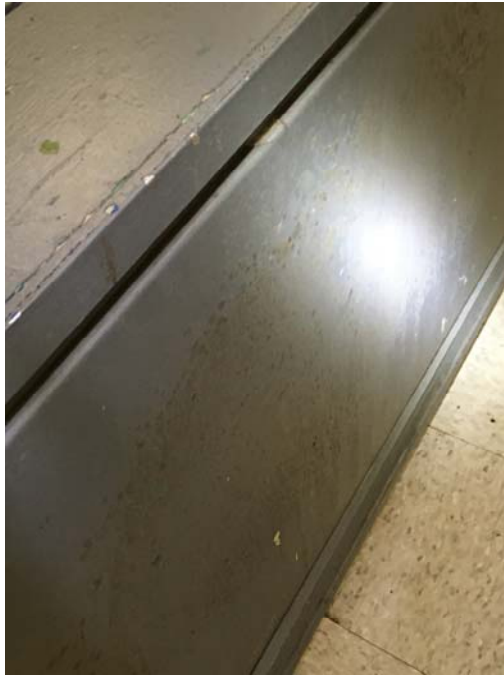
Photo 5 – Kindergarten Room 1 Mold growth was observed on the unit ventilator.
