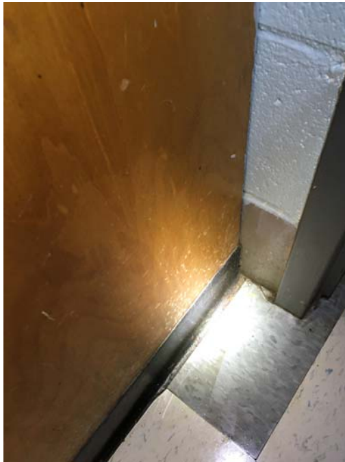
Photo 17 – Kindergarten Room 2 Mold growth was observed on the built-in wooden cabinetry and coat cubby.
